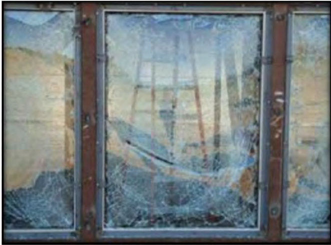
Figure C.9: Specimen 2 External Post-Blast Condition
