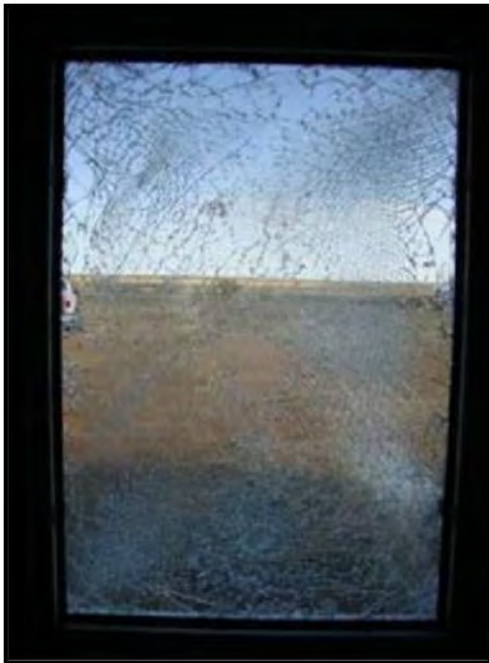
Figure C.15: Specimen 4 Internal Post-Blast Condition
