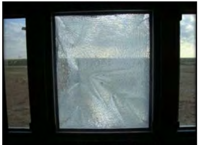
Figure C.26: Specimen 14 Internal Post-Blast Condition
