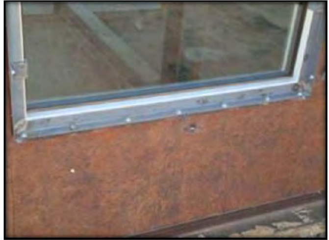
Figure C.2: L1 Bolt Connection Pre-Blast Condition
