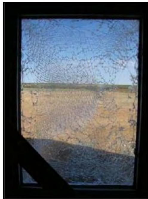
Figure C.14: Specimen 3 Internal Post-Blast Condition
