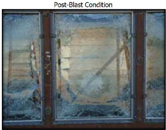
Figure C.10: Specimen 3 External Post-Blast Condition
