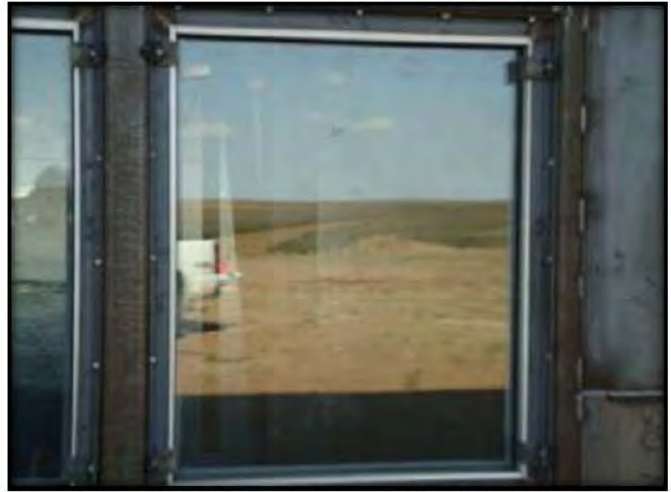
Figure C.24: Specimen 16 External Post-Blast Condition
