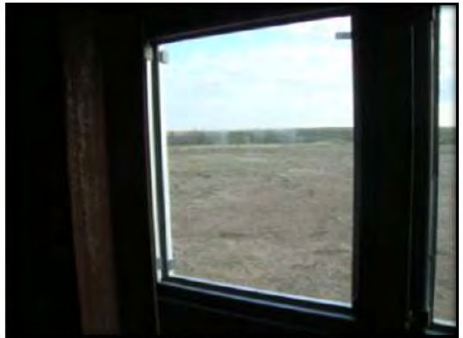
Figure C.28: Specimen 16 Internal Post-Blast Condition
