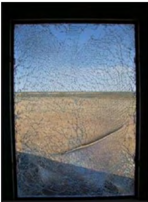
Figure C.13: Specimen 2 Internal Post-Blast Condition
